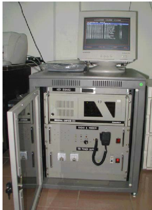
A VHF radio Sub-master Station using SM2000 FEP in a 13U height 19" equipment rack.
