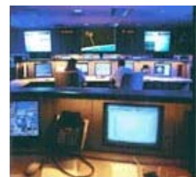
Network Control Center
