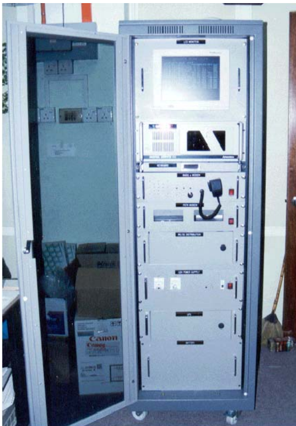
Another SM2000 FEP with VHF RTU and PSTN MODEM as communication link.
