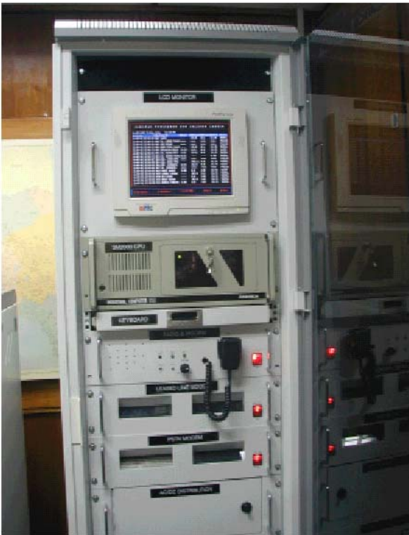
SM2000 FEP equipped with UHF Radio, PSTN MODEM, lease line MODEM, ORBCOMM satellite network as communication link to remote stations
