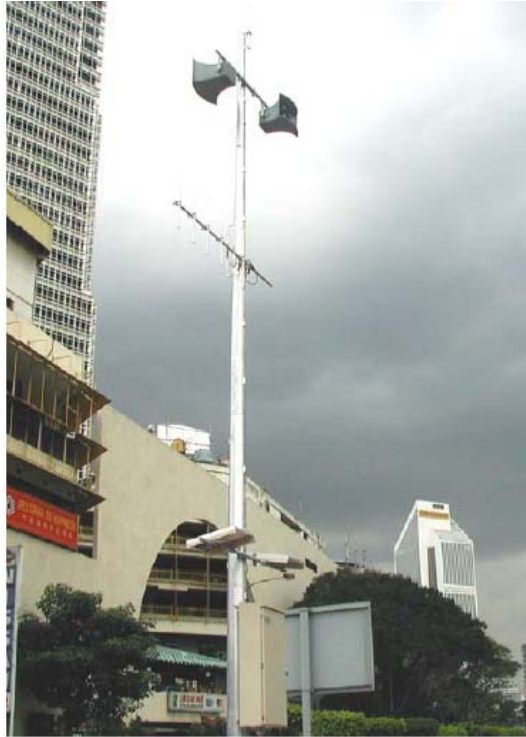
A typical siren pole with pole mounting weatherproof enclosure
