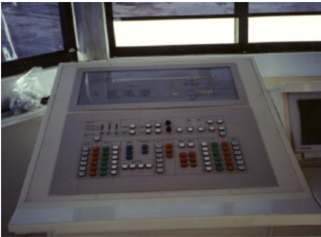
A control desk with control buttons and runway mimic
